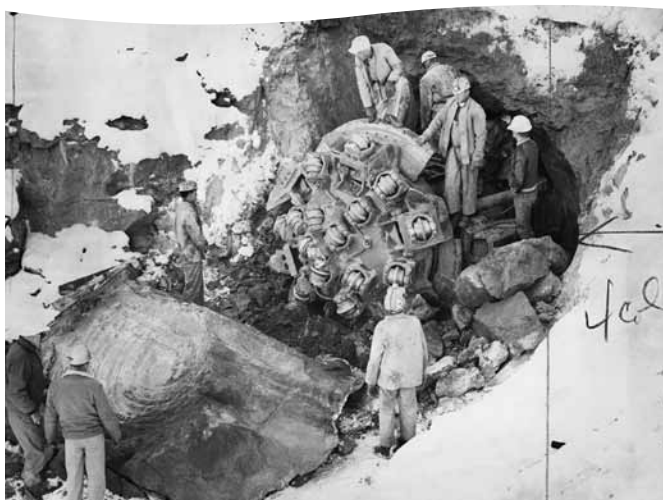
Mechanical Mole, 1971. The 80 ton machine, with its cutting face of 13 feet in diameter, drilled the Central Utah Project's Water Hollow Tunnel. When the aqueduct system was complete, it delivered water to triple the capacity of Strawberry Reservoir. Uintah County Library Regional History Center.
